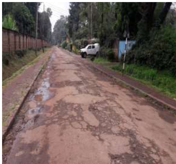
Defect: Surface failure and potholes On Kabarsiran Avenue. Date: 23.6.2020
