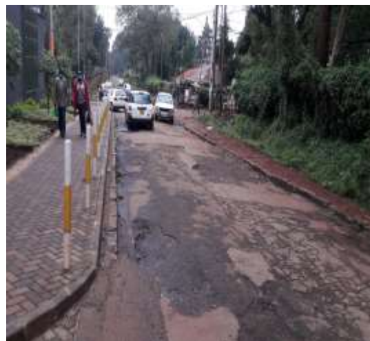
Defect : Potholes and Carriageway Base Failure due to water ponding on Kabarsiran Avenue Date: 23.6.2020
