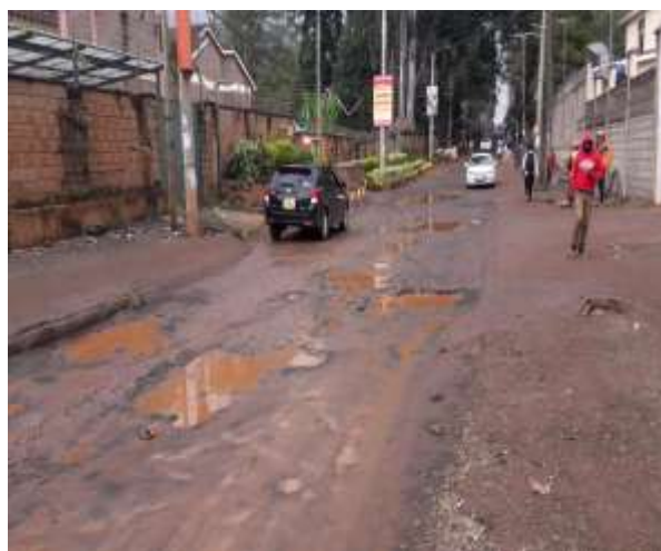
Defect: Water ponding and base failure on Musa Gitau Road Date: 23.6.2020
