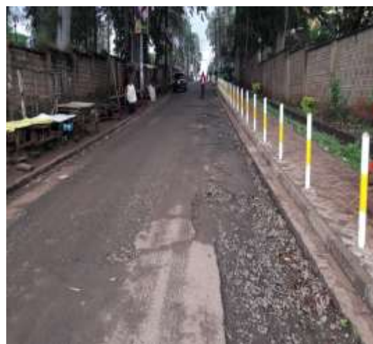
Defect: riding surface failure on Musa Gitau Road Date: 23.6.2020
