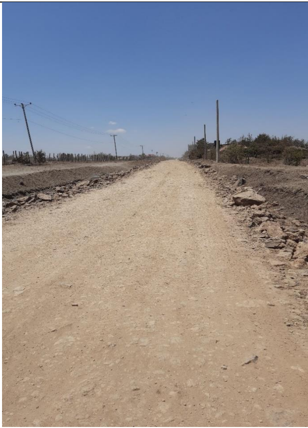
Ruts and depressions making surface uneven.
