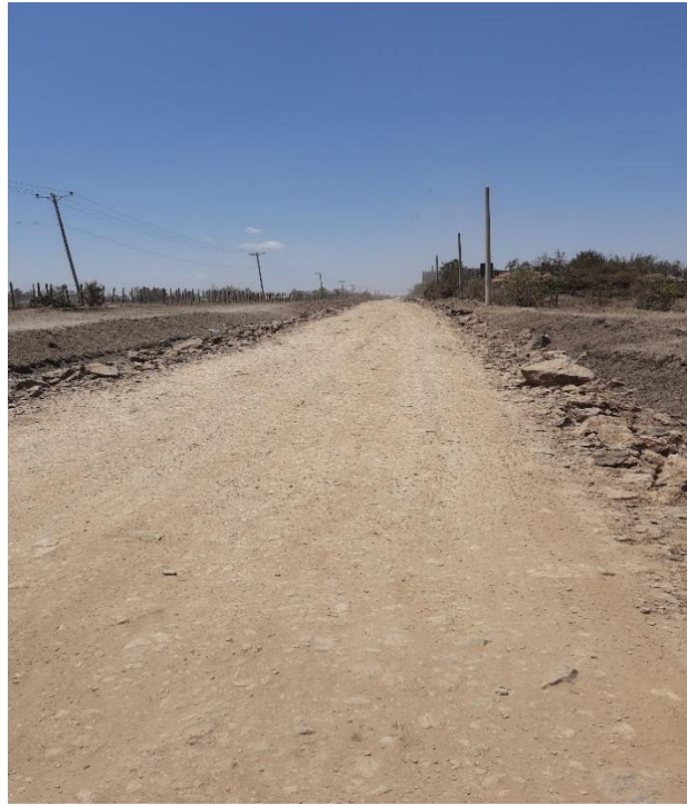
Huge boulders unsuitable as wearing course.
